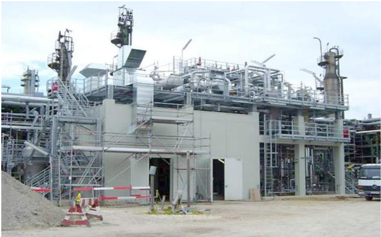
Refinery Gas Plant
