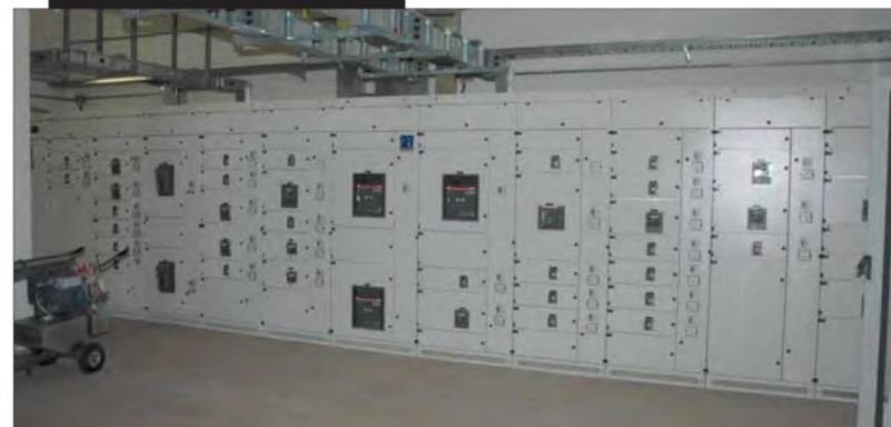
Power Center B.T. - Power Center B.T.
